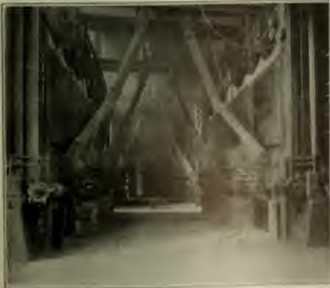
BOILER FRONTS AND STEAM
